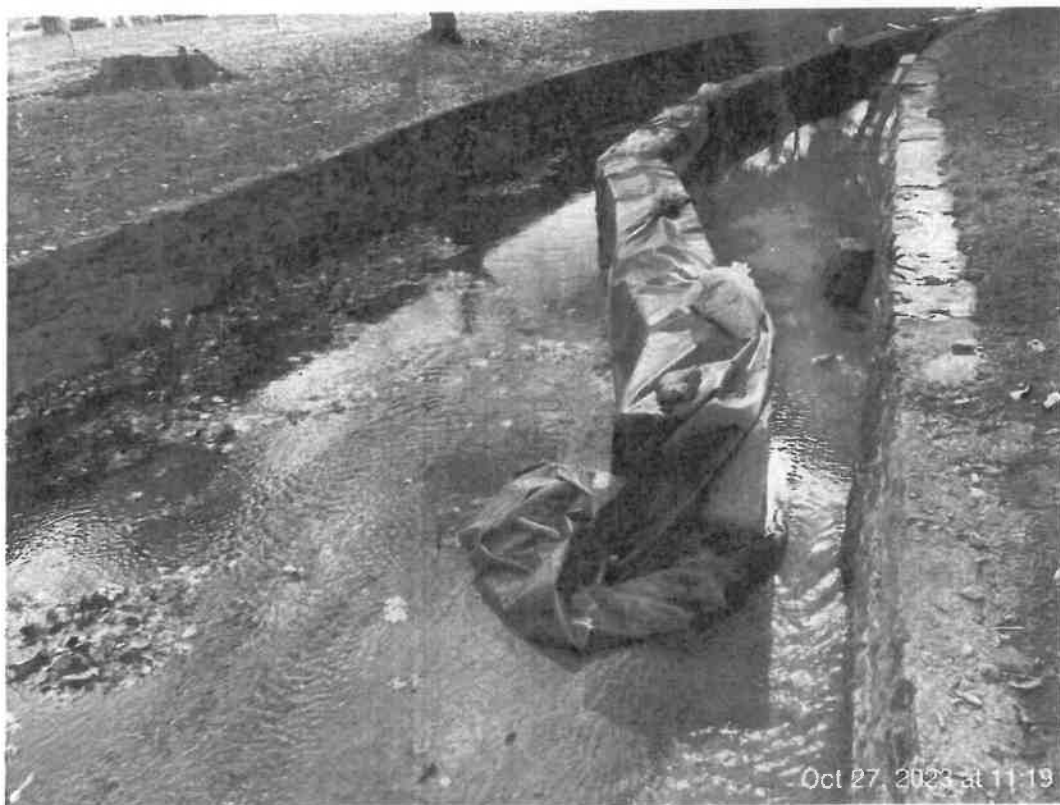
10/27/23 at 11:19AM. Sediment was flowing from construction into Warm Springs Run.
