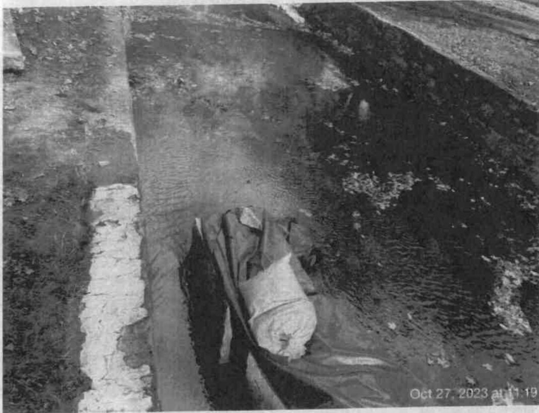
10/27/23 at 11:19AM. Sediment was discharging into Warm Springs Run.
